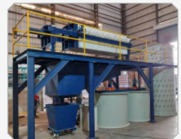
Flux Filtration System
